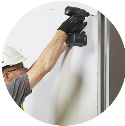
2. The wall can now be plasterboarded over the pocket and on top of the Timber Trim.
