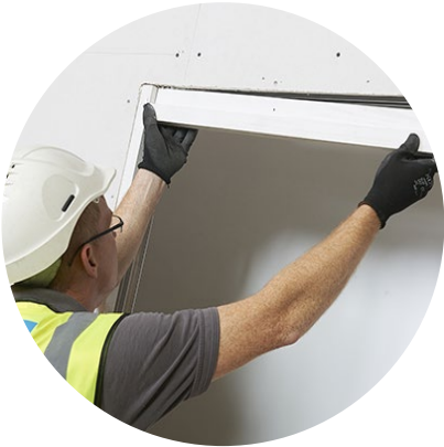
1. Install the timber head trim (before plasterboard). Cut the head trim to the opening width and slot into place.
